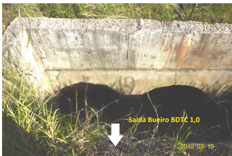
Figura 30 – BTDC 1,0 obstruindo BTTC 1,20m
